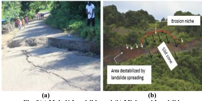
Fig. 9(a) Mahalé Landslide and (b) Miringoni Landslide
